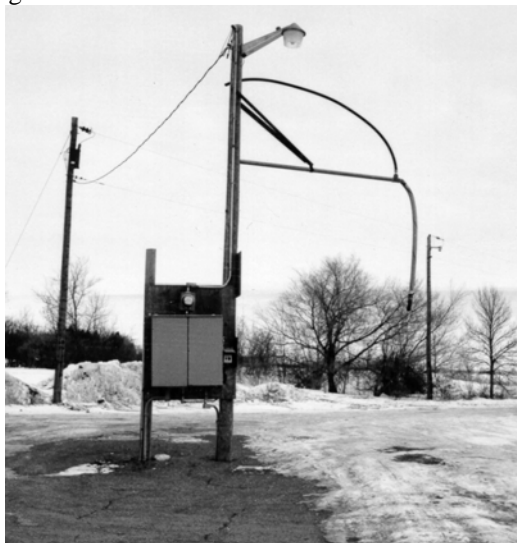
Typical community water supply.
